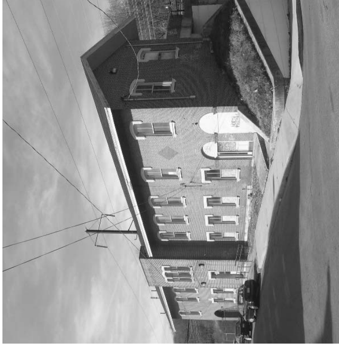
Shelter areas are in poor repair.
