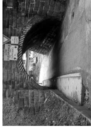
Pedestrians must walk through a very narrow and hazardous underpass.
